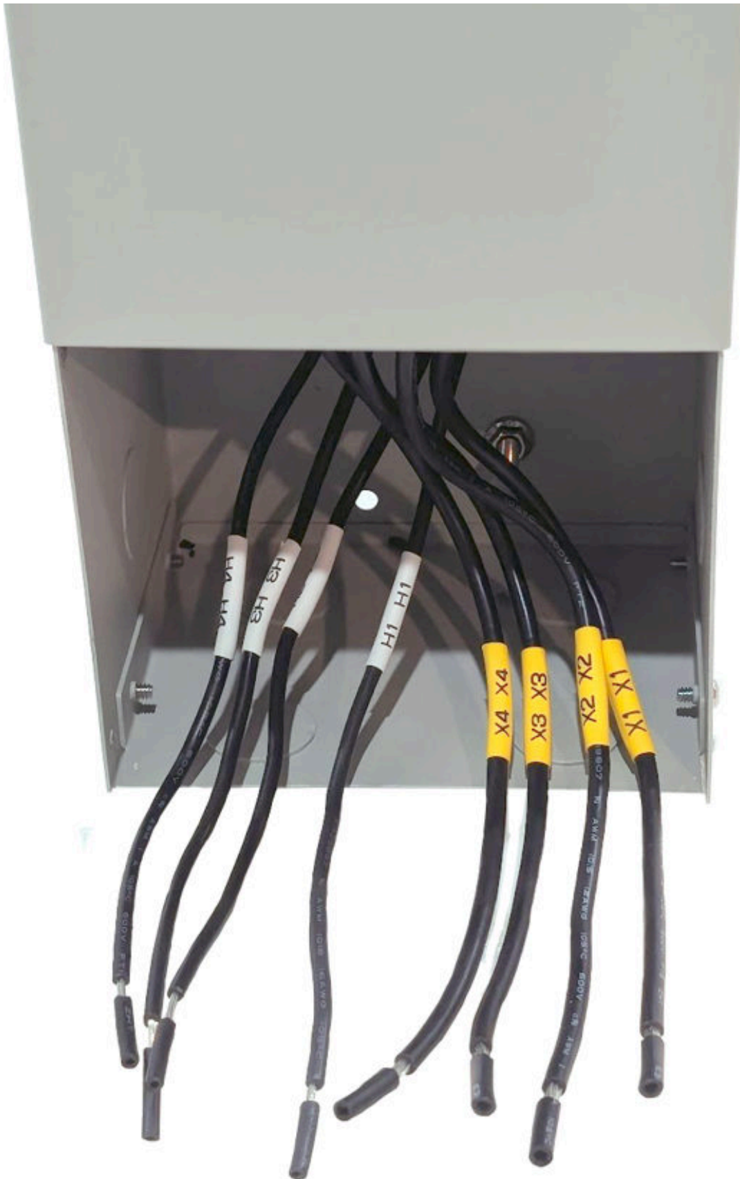
TX-A3-020K-112123 - Wiring Compartment - Primary & Secondary Leads
