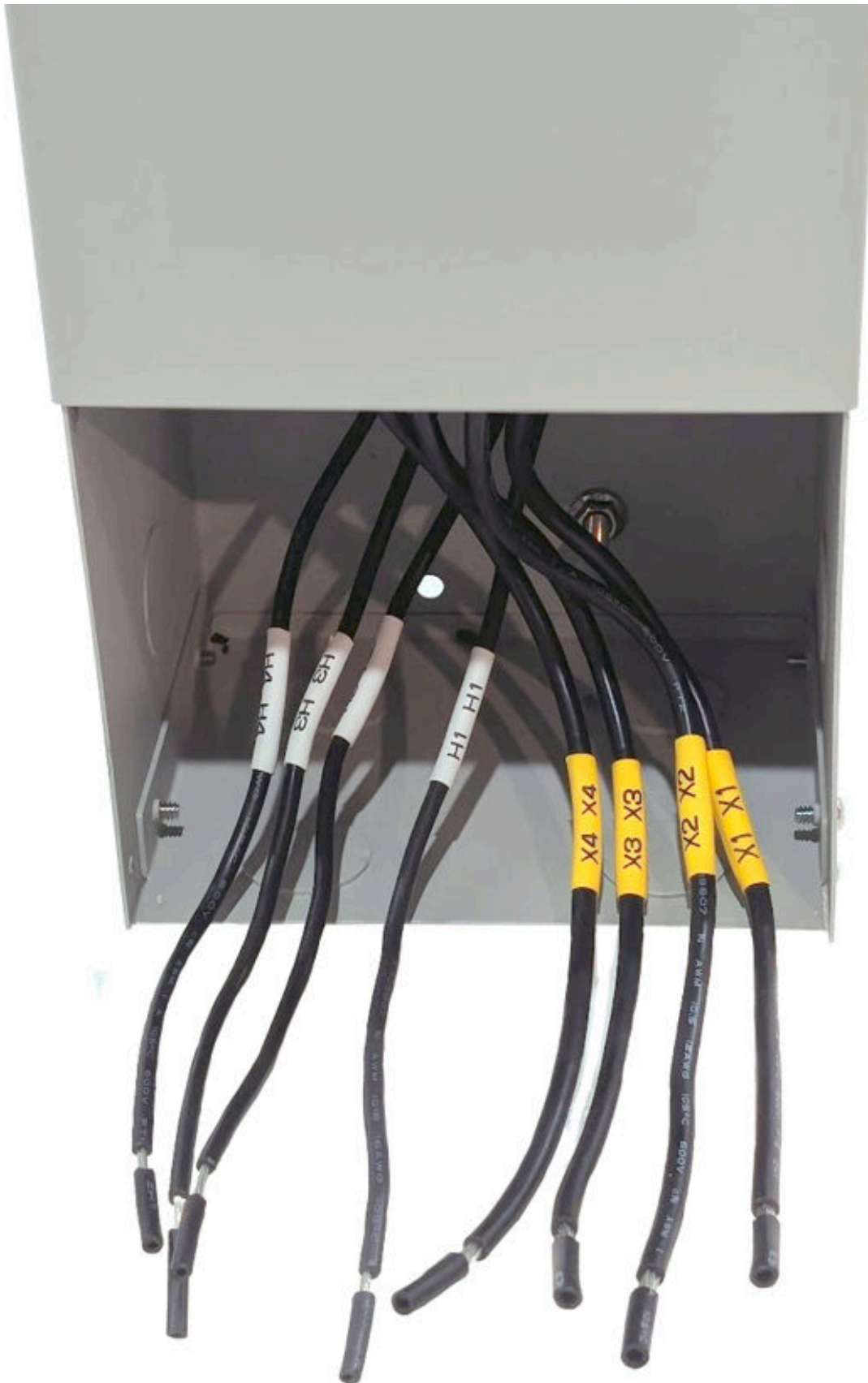
TX-A2-080H-115124 - Wiring Compartment - Primary & Secondary Leads
