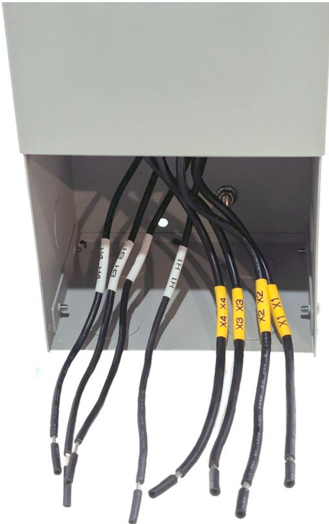
TX-A1-030H-162124 - Wiring Compartment - Primary & Secondary Leads
