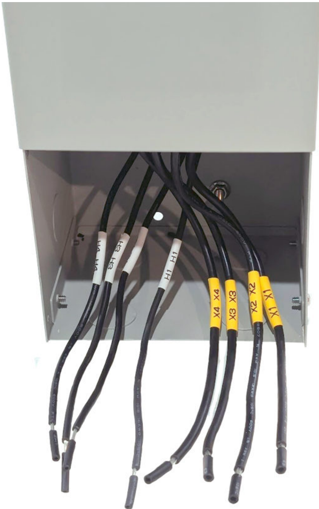
TX-A1-030H-150126 - Wiring Compartment - Primary & Secondary Leads
