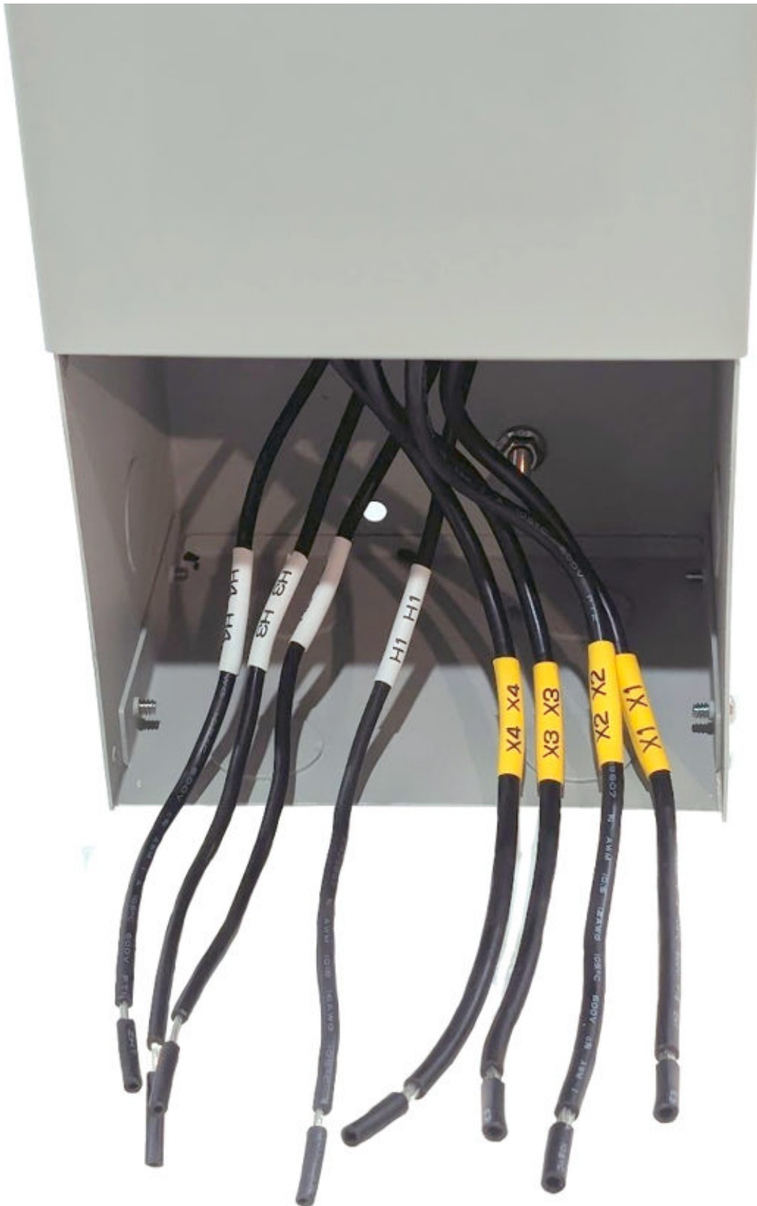
TX-A1-015H-150126 - Wiring Compartment - Primary & Secondary Leads
