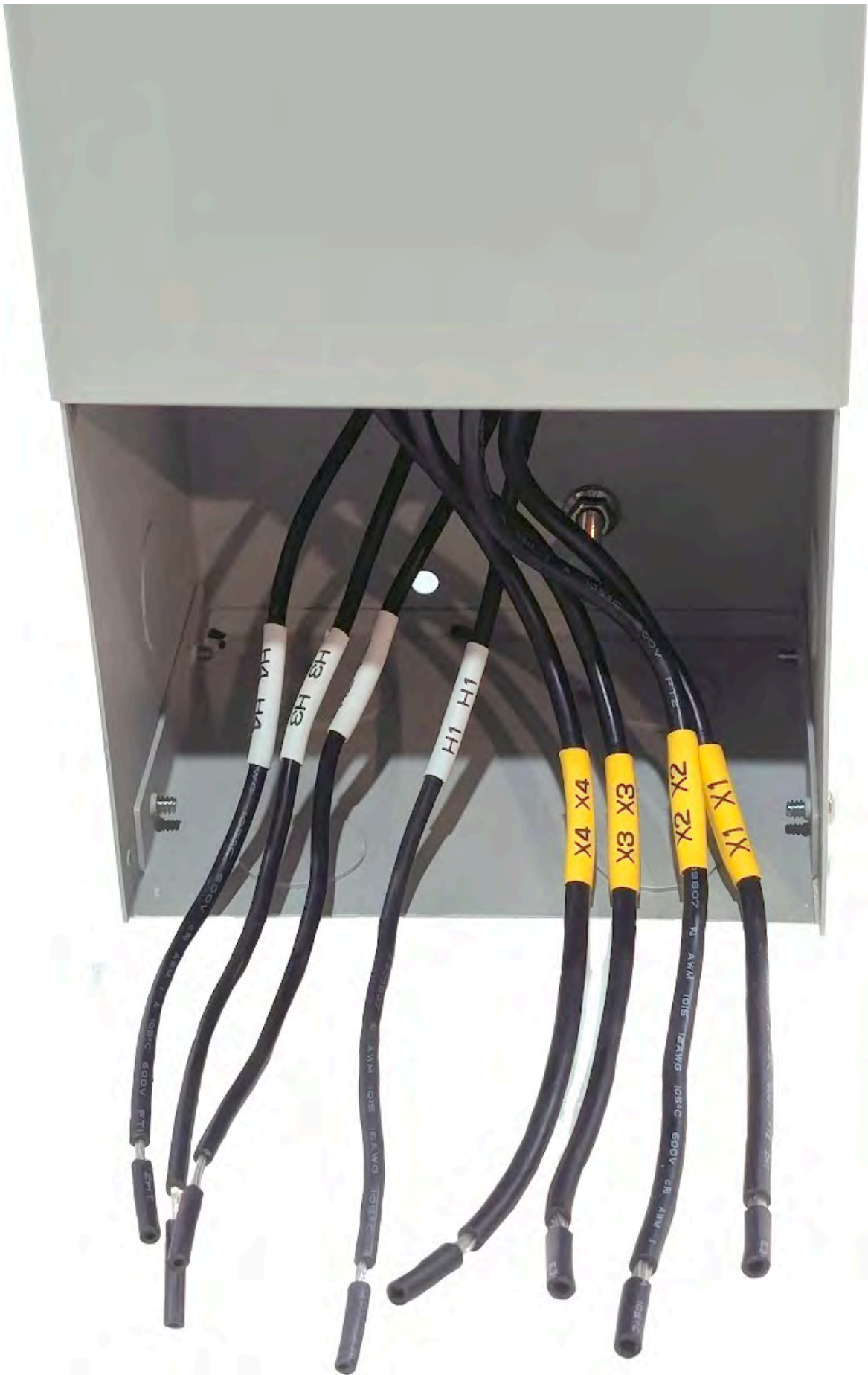
Wiring Compartment - Terminal Leads
