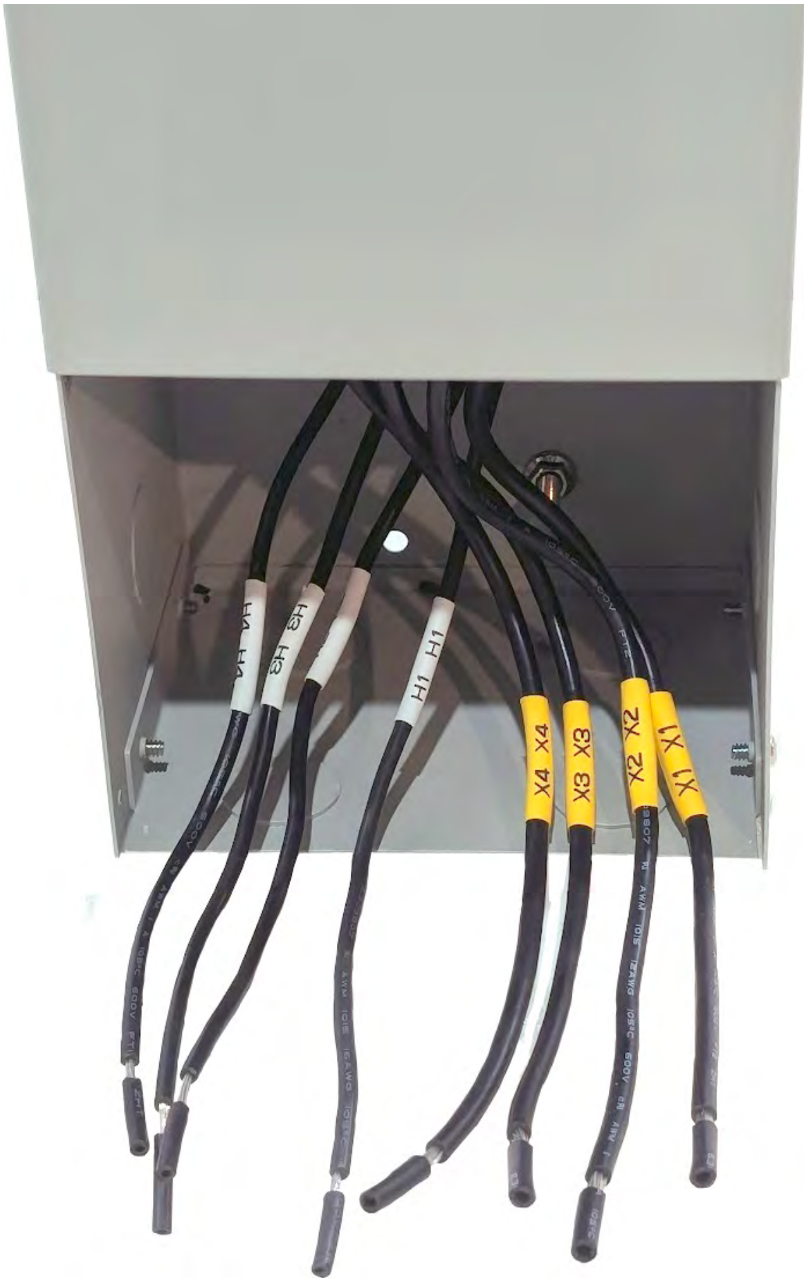
Wiring Compartment - Terminal Leads
